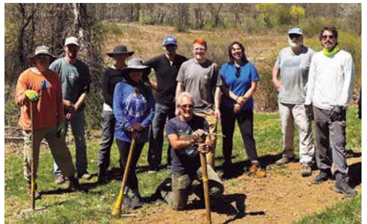
SRA Volunteer Work Party initiating construction of Hillside Farm Trail in April 2023.
